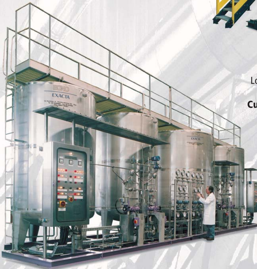
Jebel Ali "G" Power and Desalination Plant - United Arab Emirates Antifoam and Antiscale Dosing Package. Customer: Weir Westgarth - Scotland
